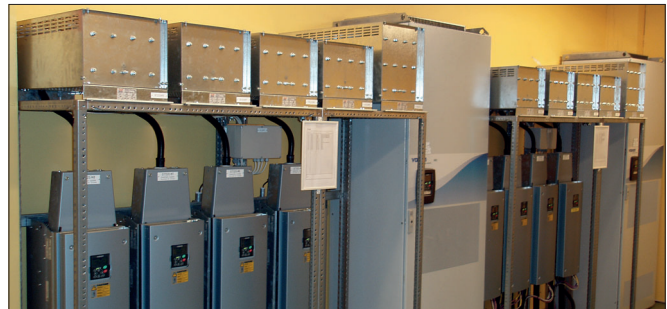
Cressall DBR Series braking resistors installed on a shelf above the AC variable speed drives at a paper mill.
